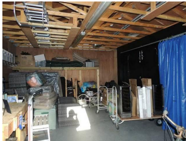
Interior of the garage. Note lack of features that might be occupied by bats
