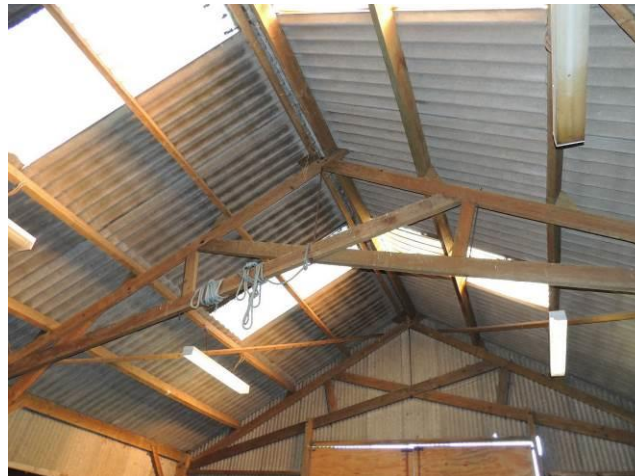
The interior of the workshop had no features that might be occupied by bats
