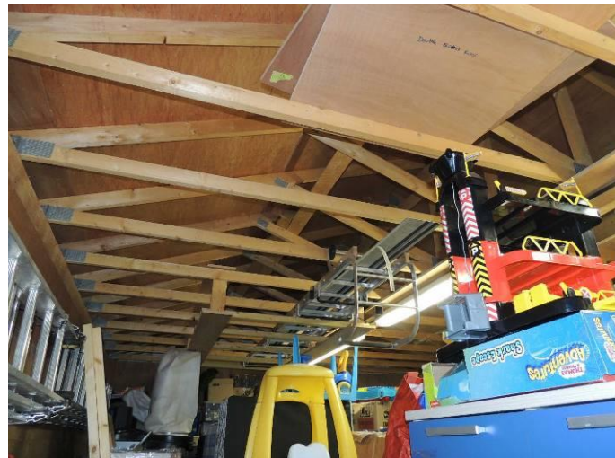
Interior of the garage. Note lack of features that might be occupied by bats
